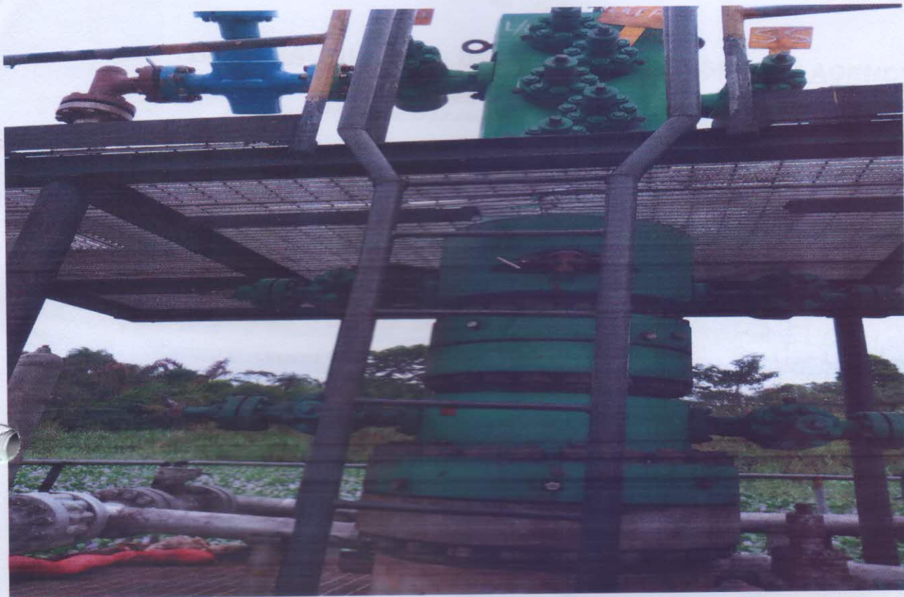
The well head where the SSV Failed.
